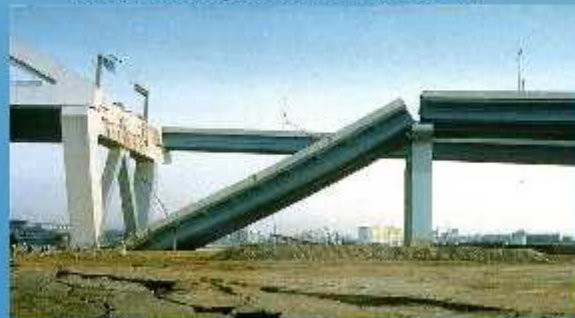
Failures of structure caused by loss of strength of underlying soil
